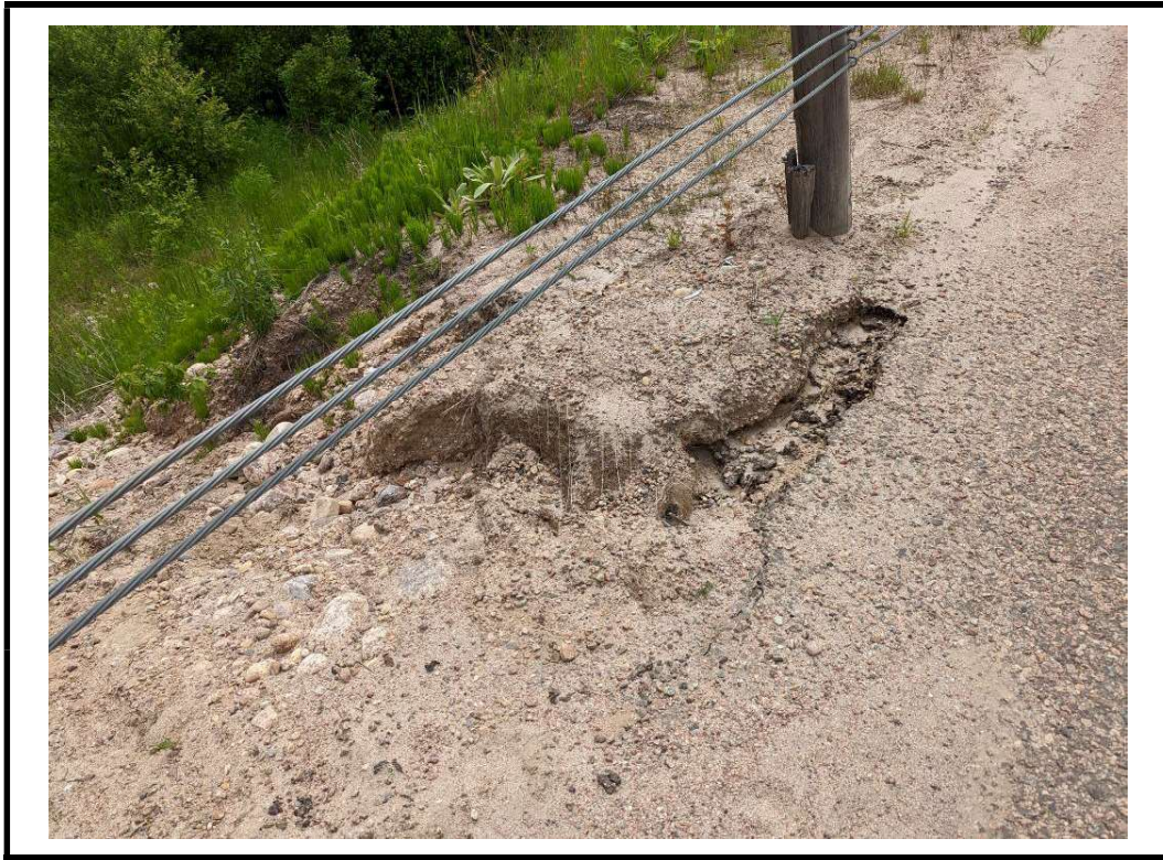
Photo 11 Heavy washout noted at southwest corner over structure
