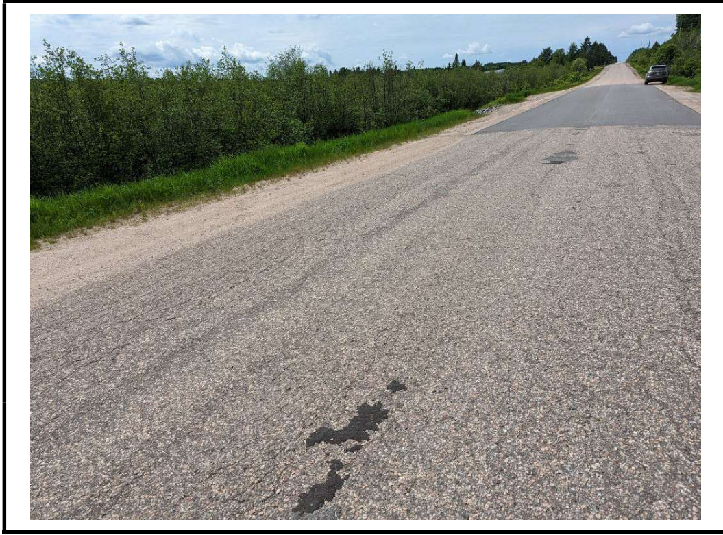
Photo 7 Medium to wide longitudinal cracks and patches noted at east approach
