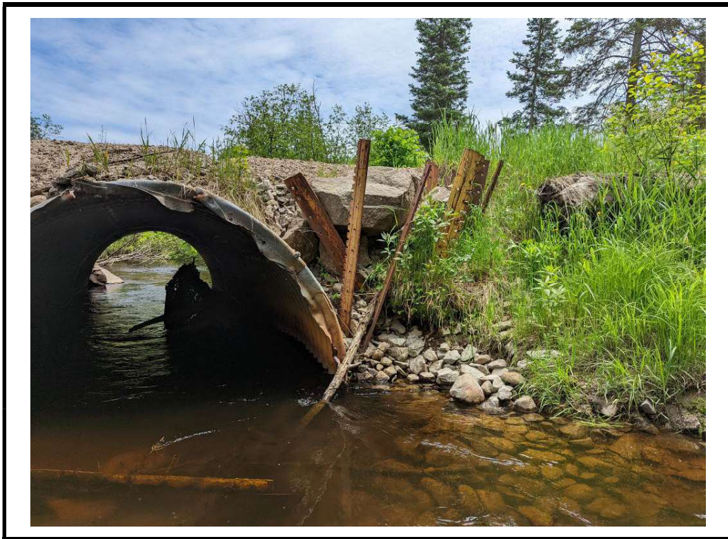
Photo 8 Dents noted at west end of barrel
