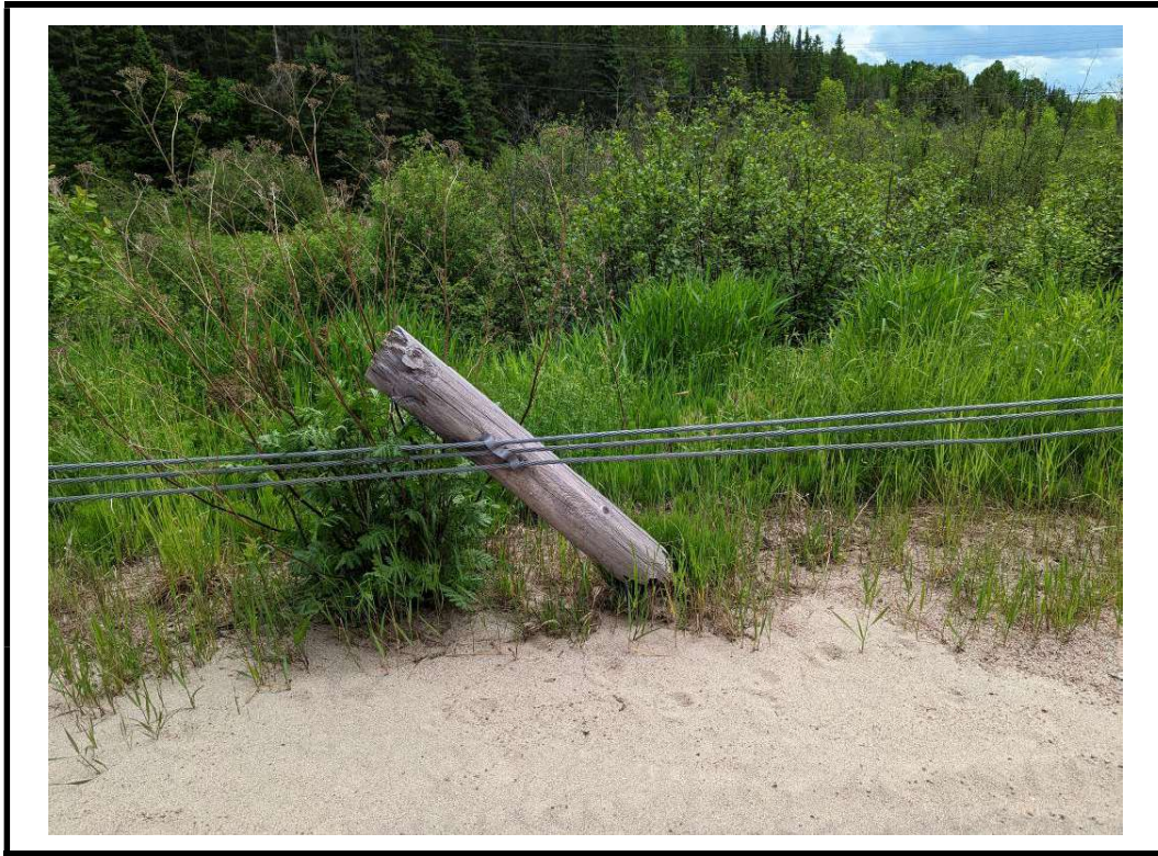
Photo 7 Broken post observed in north barrier
