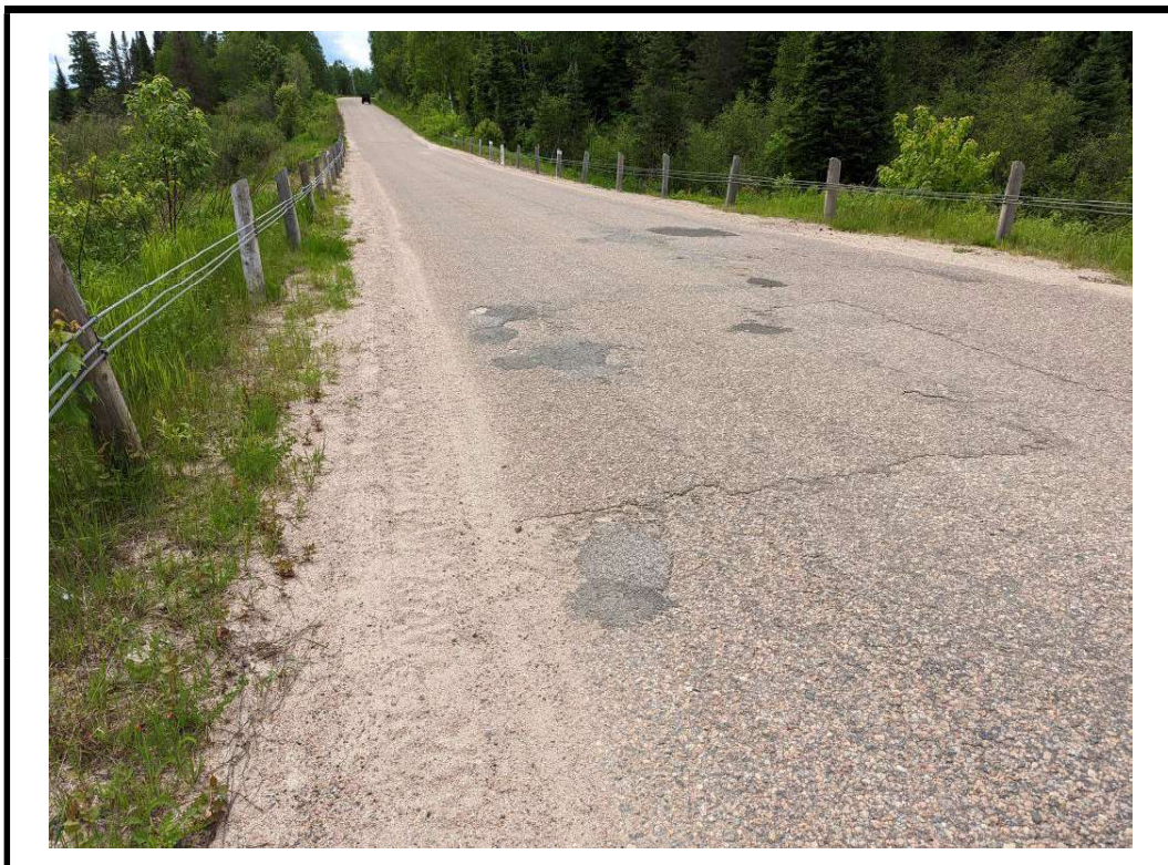
Photo 8 Moderate raveling, patched potholes noted in east approach wearing surface
