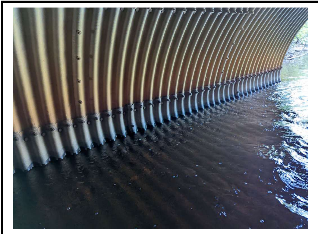
Photo 8 Light to moderate corrosion noted at waterline
