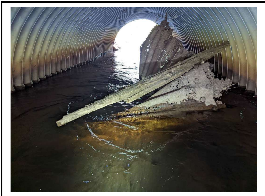
Photo 12 Damaged section of CSP in barrel, does not appear to be from this structure
