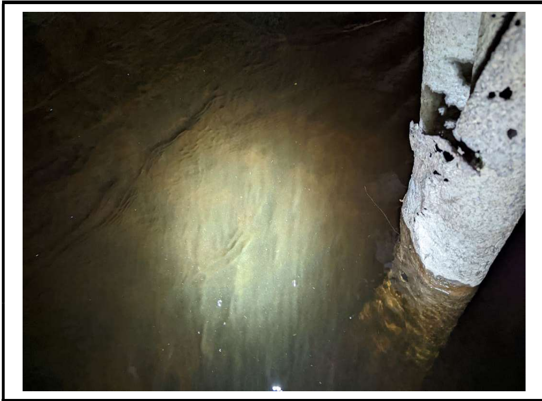
Photo 11 Severe perforation noted at and below waterline
