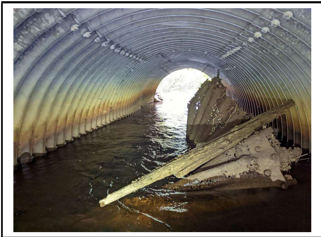
Photo 10 Efflorescence noted at seams and along boltline
