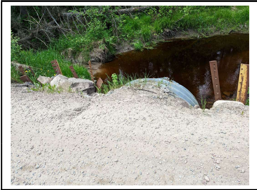
Photo 7 Erosion of edge of shoulder at west end of structure
